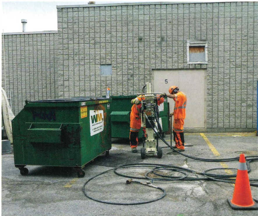
Direct injection of solutions of ISCO reagents to the subsurface using drilling equipment and low pressure pumping system.
